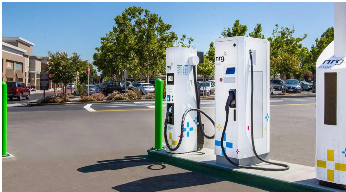
Figure 5: Example of Battery Electric Vehicle Chargers
